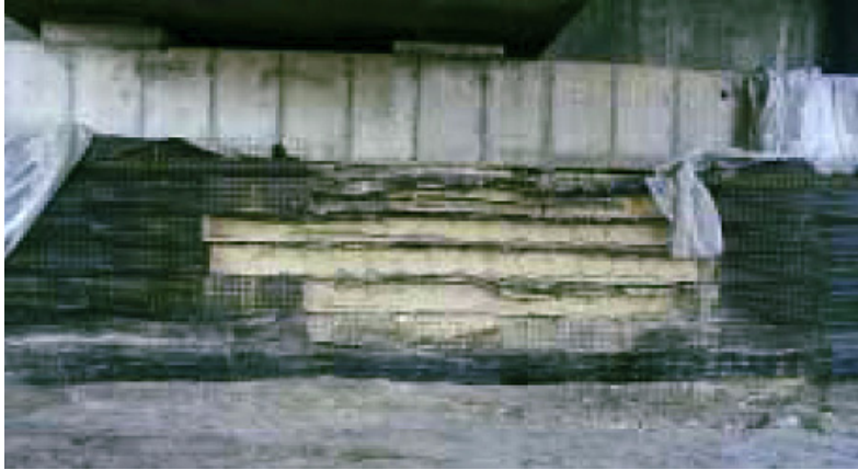
Figure 30, Fire Damaged Reinforcement
