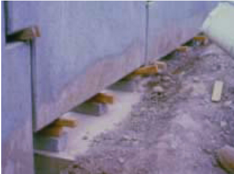
Figure 2,Improper Leveling Pad
