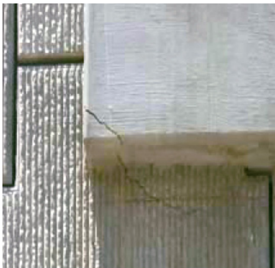
Figure 18, Cracked Panel and Cheek Wall
