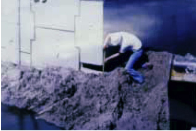
Figure 25, Settlement from Excavation
