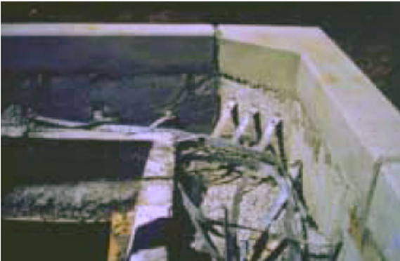
Figure 24, Not properly avoiding drainage structure
