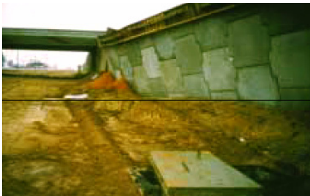
Figure 27, Wall Failure from Exterior Excavation
