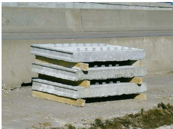
Figure 8, Proper Panel Storage
