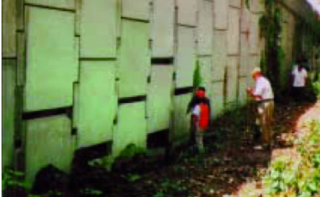
Figure 28, Settlement from a leak in a pipe joint
