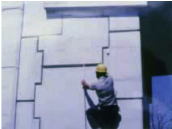
Figure 26, Joints Opening from Settlement
