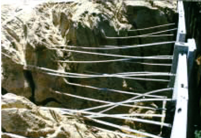
Figure 22, Wash Out From Around Reinforcement
